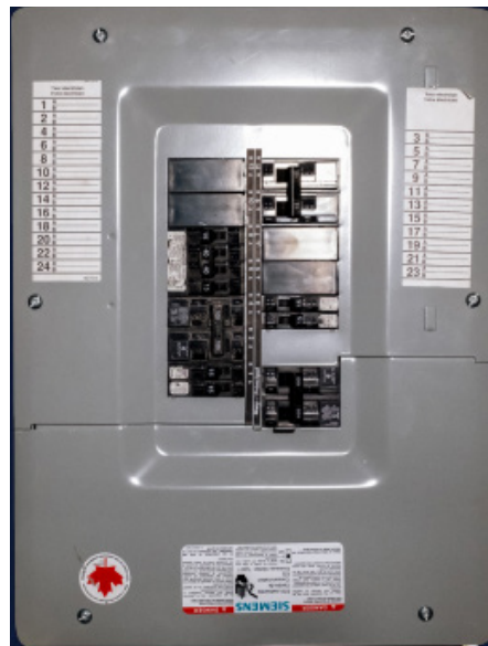
BusGuard with the Panel cover on
